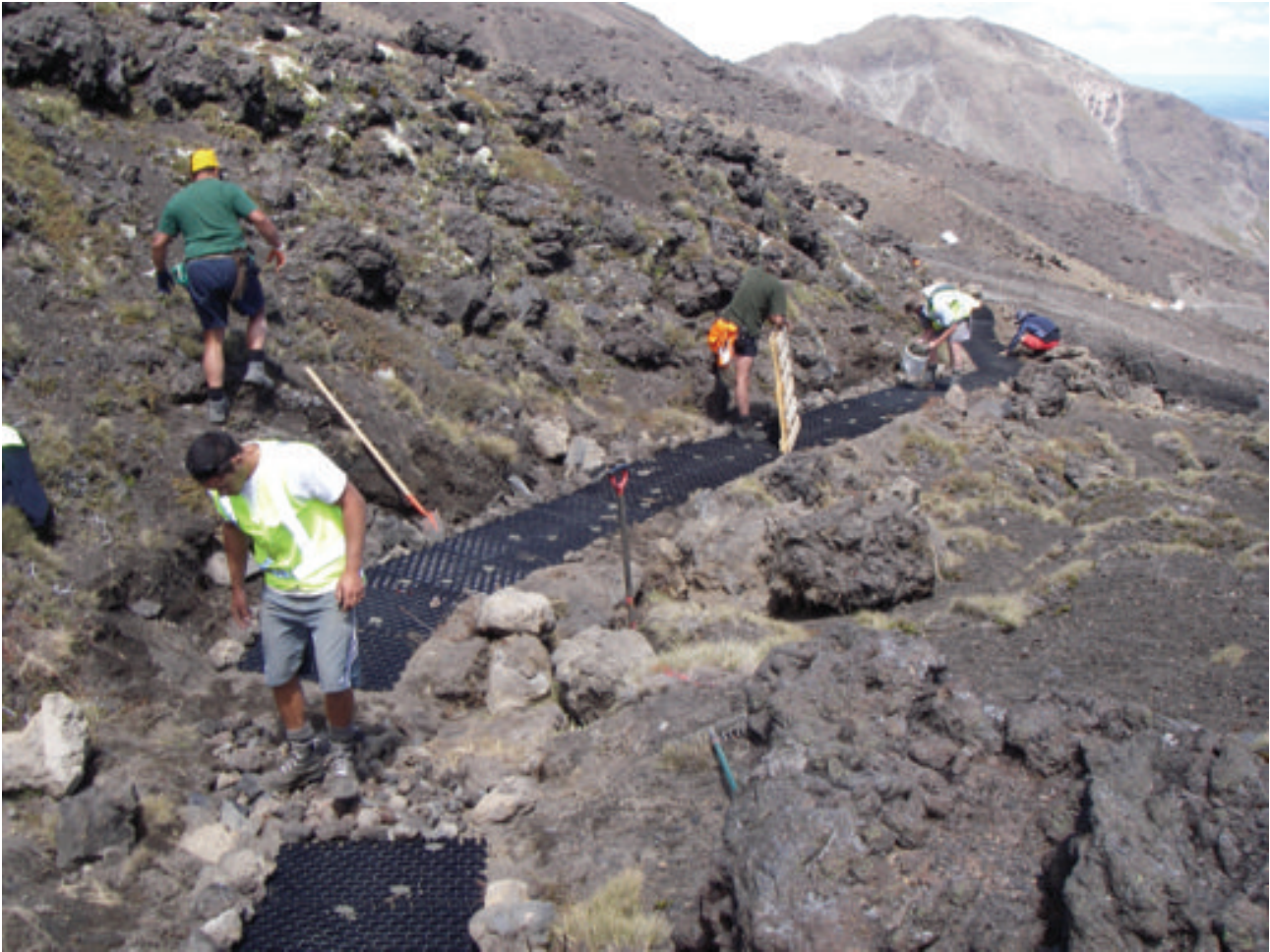
Above: Contractors “Logic Forest Solutions” working on the deviation laying Jakmat to form a stable base for the new track. Photo: John Wilton
