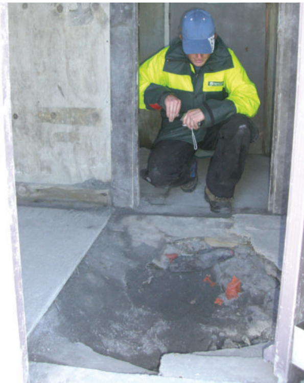
Above: Ian McNickle (DOC) surveys the hole caused by the blast of the 25 September eruption in the floor of the Dome Equipment Shed. Photo: Harry Keys
