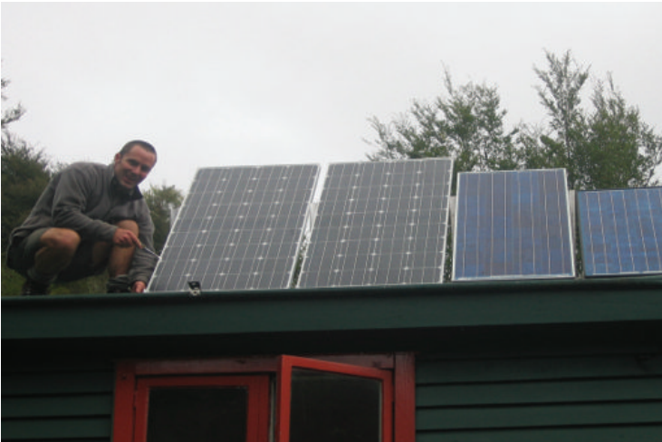
Above: Nathan Walker makes some last minute adjustments to the solar panels on the new Te Whaiiau trap accommodation. Photo: Julie Greaves
