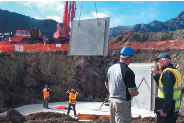
Above: Consultant Engineer Ian Smith oversees the placement of panels for the buffer tank on the Whakapapa Ski field . (Photo: Warren Furner)
