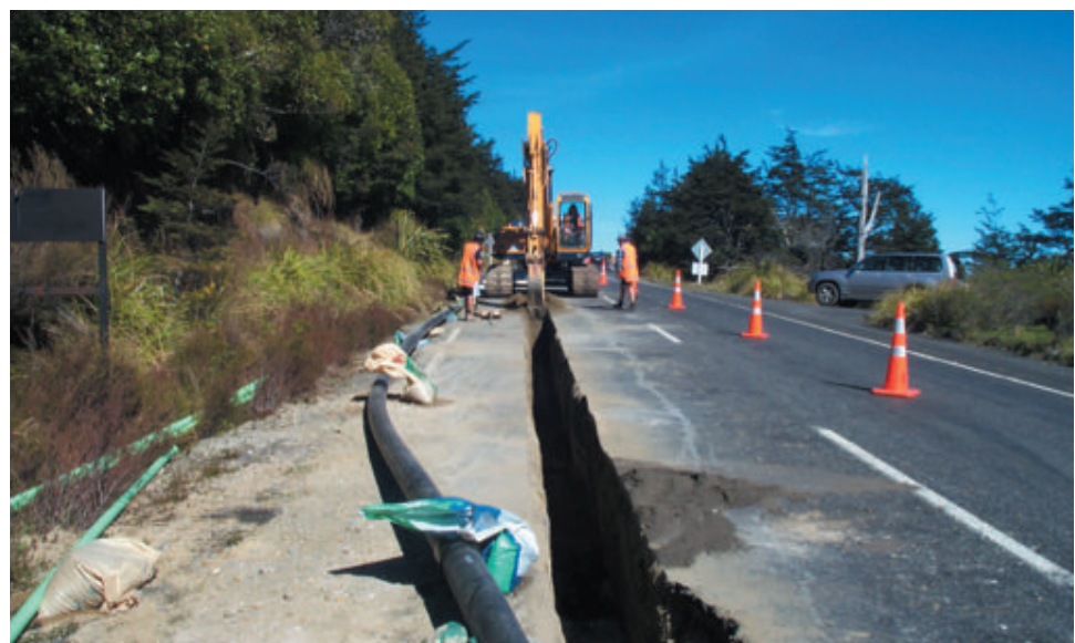
Right: The shoulder of the Bruce Road was used to lay the sewerage pipeline from Iwikau to Whakapapa. (Photo: Warren Furner/DOC)
