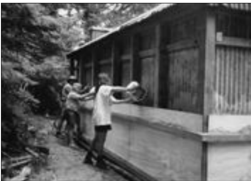
Above: DOC staff and Tongariro Natural History Society volunteers refill the rebuilt wall of Waihohonu Historic Hut with the original pumice insulation removed during the restoration. (Photo: John Newton)
