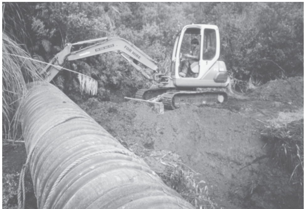
The little digger that could. Repair work being undertaken on a section of the 42 Traverse in Tongariro Forest. (Photo: Barbara Curtis)
