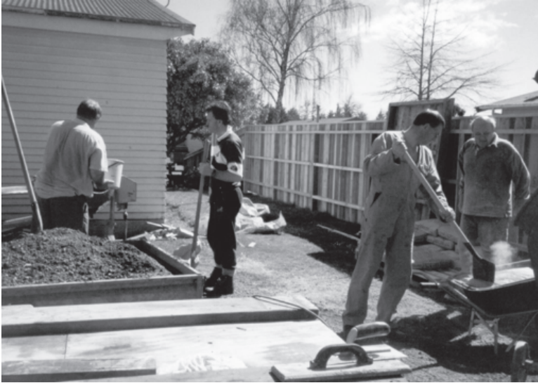
DOC staff volunteered their time to help complete several project Hemi Kingi had underway before his death, including a driveway and paths. (Photo: Herwi Scheltus)
