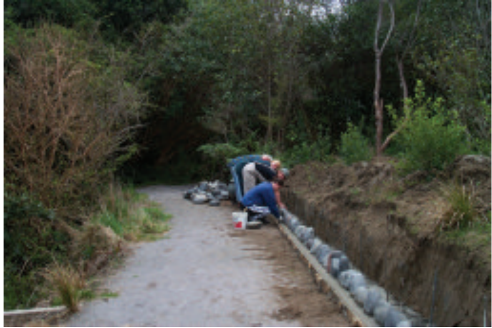
Conservancy staff from Kaupapa Wahine building a stone wall as part of the redevelopment of the Tongariro National Trout Centre. (Photo: Maureen Smith)
