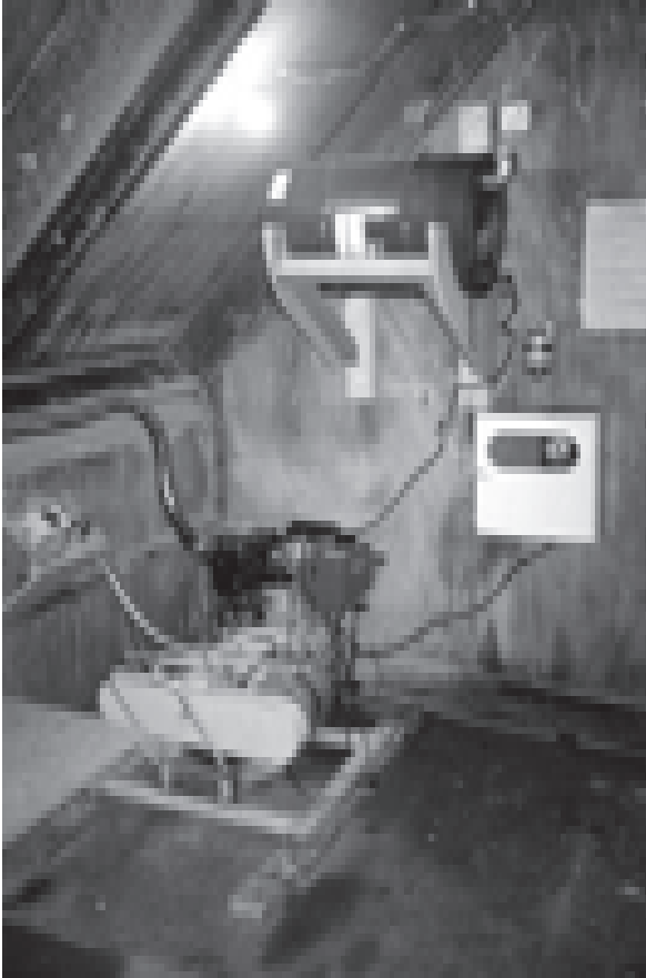
Photo of Dave Rothchild's new charging system inside Dome Shelter. The system which uses a diesel generator (bottom left) seems foolproof, and as yet no-one who has tried to start it has failed. (Photo: Harry Keys)
