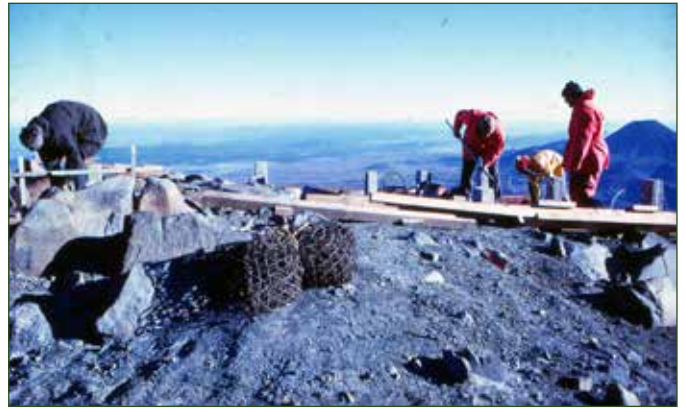
1976 preparing foundations for the Glacier Knob Shelter 700m north of the Crater Lake. It's primary purpose was to house volcanic warning equipment away from the Crater Lake. Photo: Pat Sheridan
