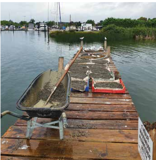
Construction of nesting areas on the Motuoapa jetty. These areas quickly became hot real-estate once the pontoons were towed.
