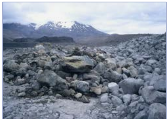
Figure 3. Bund during construction showing boulders in the sacrificial apron on left and the main bund on the right, before the cover layer was added.
