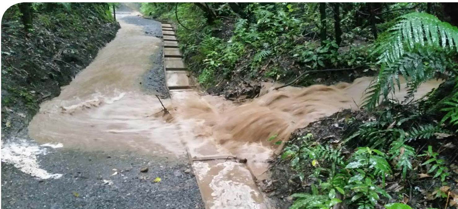
Figure 3: Distributary overflow overwhelming a box culvert on the TAC after heavy rain on 12 April 2017. Photo: Ben Scrimgeour
