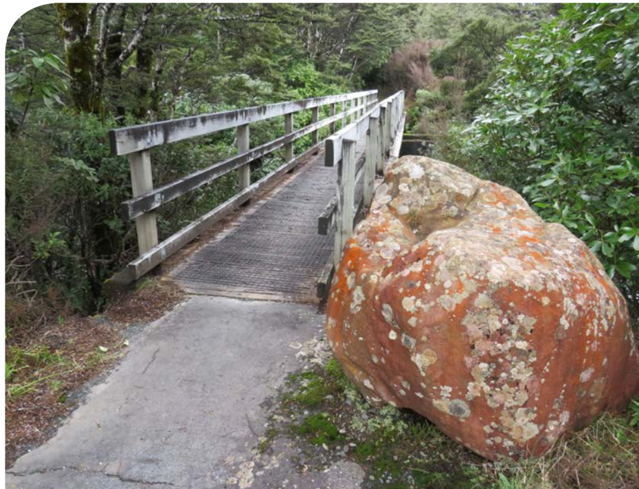
Above: Bridge over the Whakapapanui Stream. Left: Start of the Whakapapanui Track. Photos: Stacey Faire
